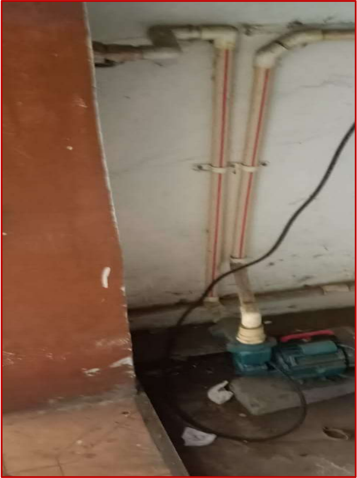
Out let pipe from RO plant connected to garden
